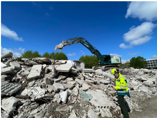
Fig 8: Genbrugsbetonen til mockuppen stammer fra Kingo Karlsens nedrivningsarbejde i Gellerupparken. / The reused concrete for the mockup is sourced from the demolition work in Gellerup by Kingo.
